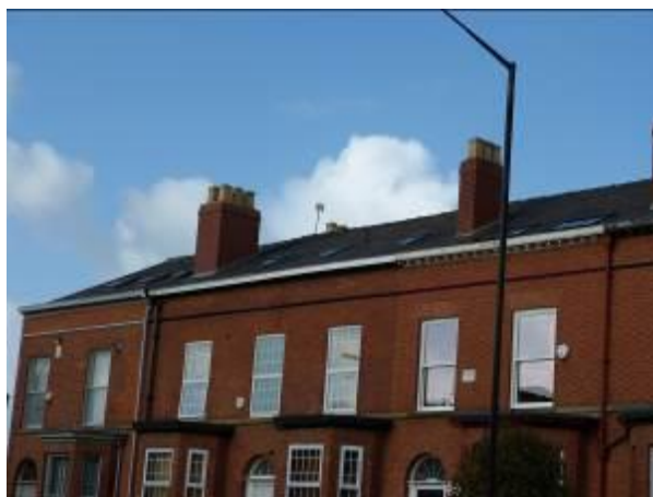
UPVC windows in mock Georgian (multi-paned) and Victorian (sheet glass) windows, with different sized roof lights above
