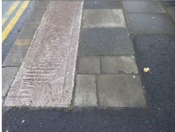
Uneven pavement surface on Chester Road
