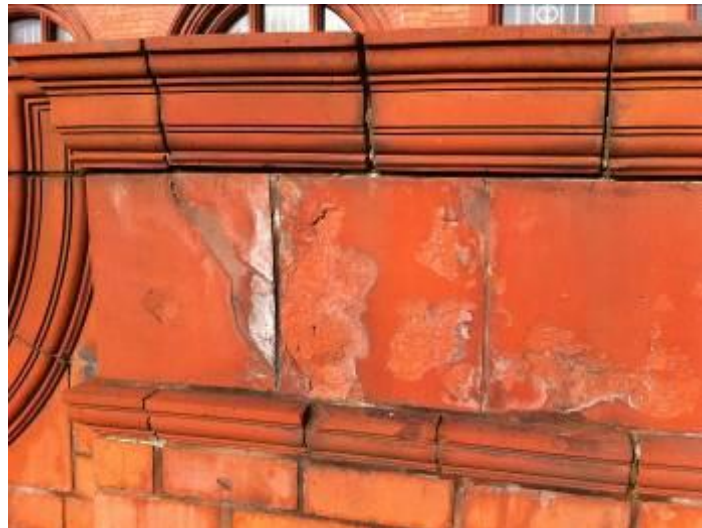
Damaged terracotta blocks to the boundary wall
